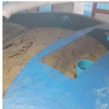
KITCHEN WASTEWATER TANK
